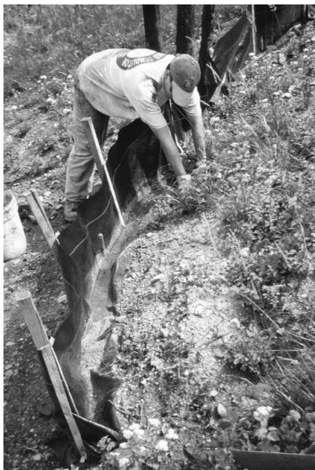
Fig. 3. Typical sediment fence where accumulated sediment is being removed.
