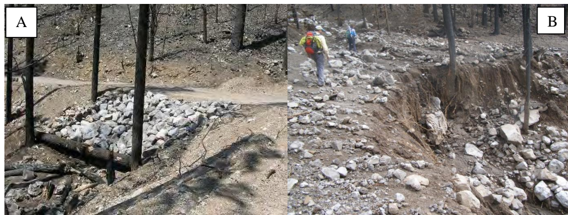
Figure 1. Rock armoring along the Waterline Road before (A) and after (B) the July 20 th flood.
