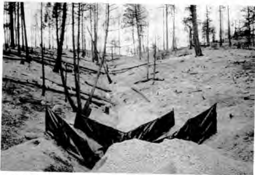
Fig. 2 Photo from summer 2003 showing a pair of sediment fences, the piles of sediment excavated from the fences, and the relatively bare hillslopes one year after the June 2002 Hayman Fire.
