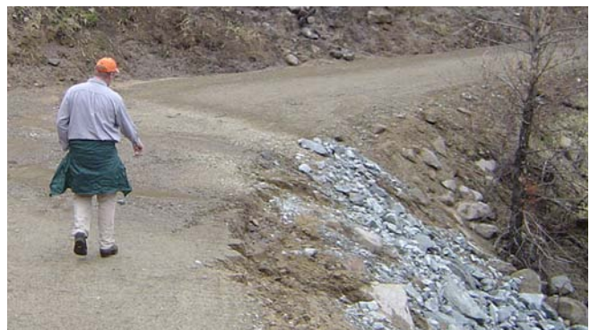
The collection point of a rolling dip with a road fill slope (an area where collected water will drain) and armored with rock after the 2007 Tripod Fire in Washington.
