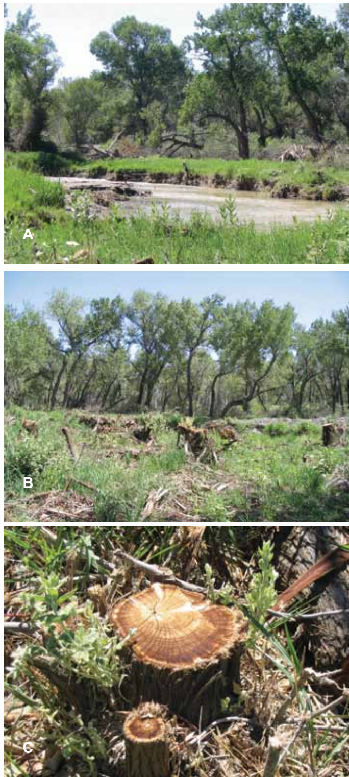
Figure 33 —Area along the Shoshone River that had been mechanically treated (2009; excavator-mulcher) to control Russian olive (A,B). Following mechanical treatments, Russian olive stumps were individually treated with an herbicide (triclopyr®) penetrating oil mix to kill the tree; however, many stumps resprouted (B).
